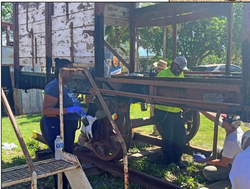
Left: Neeshell got going on the “French” side sill and door track while Ryan took over the middle. Derrick drew one of the short straws, this time working on the bottom of the sills.
